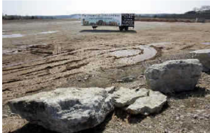
Ground has been broken for The Shoppes at Vista Lontana, south of downtown Lake Ozark. It will have upscale shops and office space, and will be adjacent to 180 luxury lakeshore condominiums under construction on the 30-acre site.
